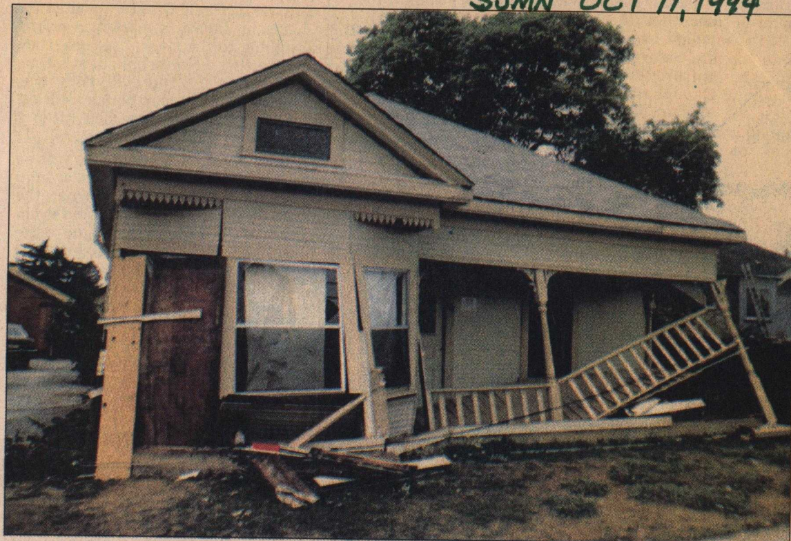
Many older houses in Watsonville were wrenched off their foundations by the force of the quake.
