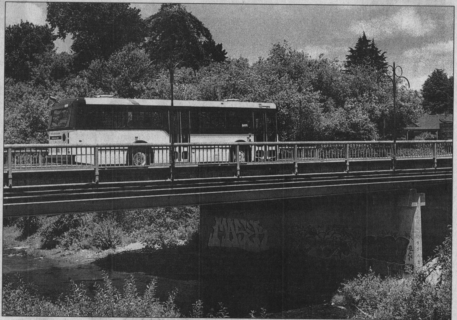
Bargetto Bridge, which crosses Soquel Creek in Soquel Village, will be replaced by one with fewer center supports.
