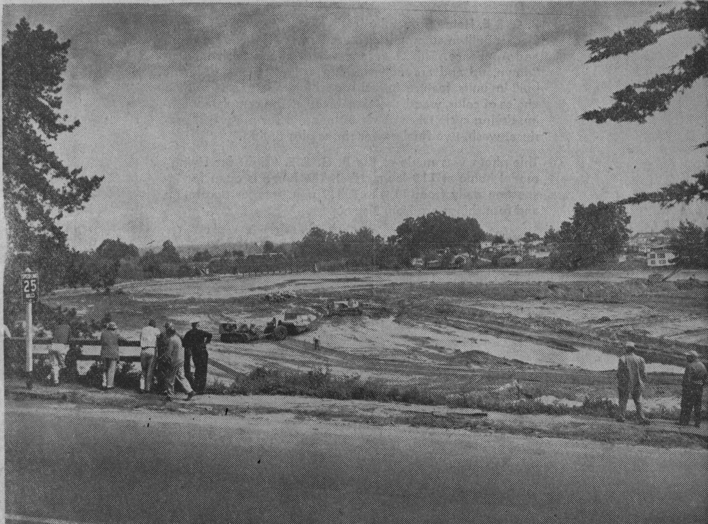
Lake-side superintendents watch as monster bulldozers cross and criss-cross the drained bed of Wood's lagoon in Twin Lakes. To be converted to a 320-boat small craft harbor, construction of jettys will commence soon for the $3.7 million project.
