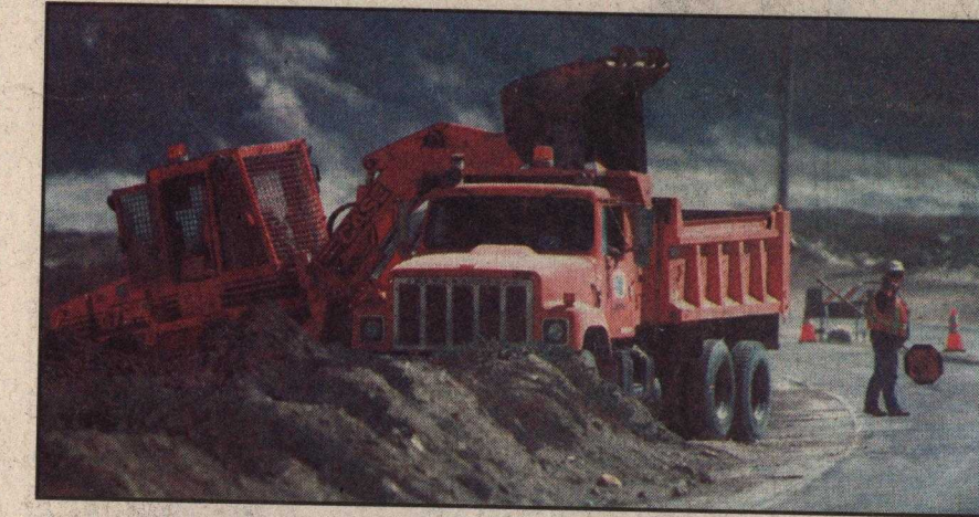
Caltrans worked along Highway 1 near Waddell Creek last week to remove accumulated debris from the base of large cliffs next to the roadway.
