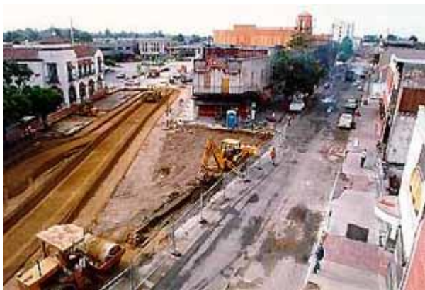
This photograph shows the Flatiron during the reconstruction following the 1989 Loma Prieta earthquake. The Flatiron itself was later demolished because of earthquake damage. The red and white sign on the building said "Teacup," which was the name of the Chinese restaurant and bar.
