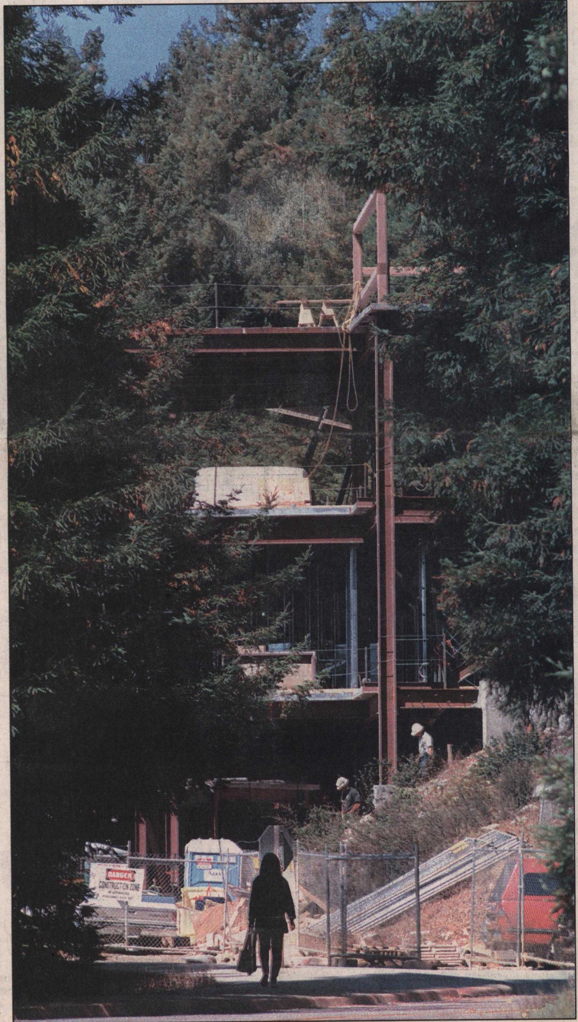
Going up: Construction in front of the Bay Tree bookstore at UC Santa Cruz is scheduled to be completed in spring.
