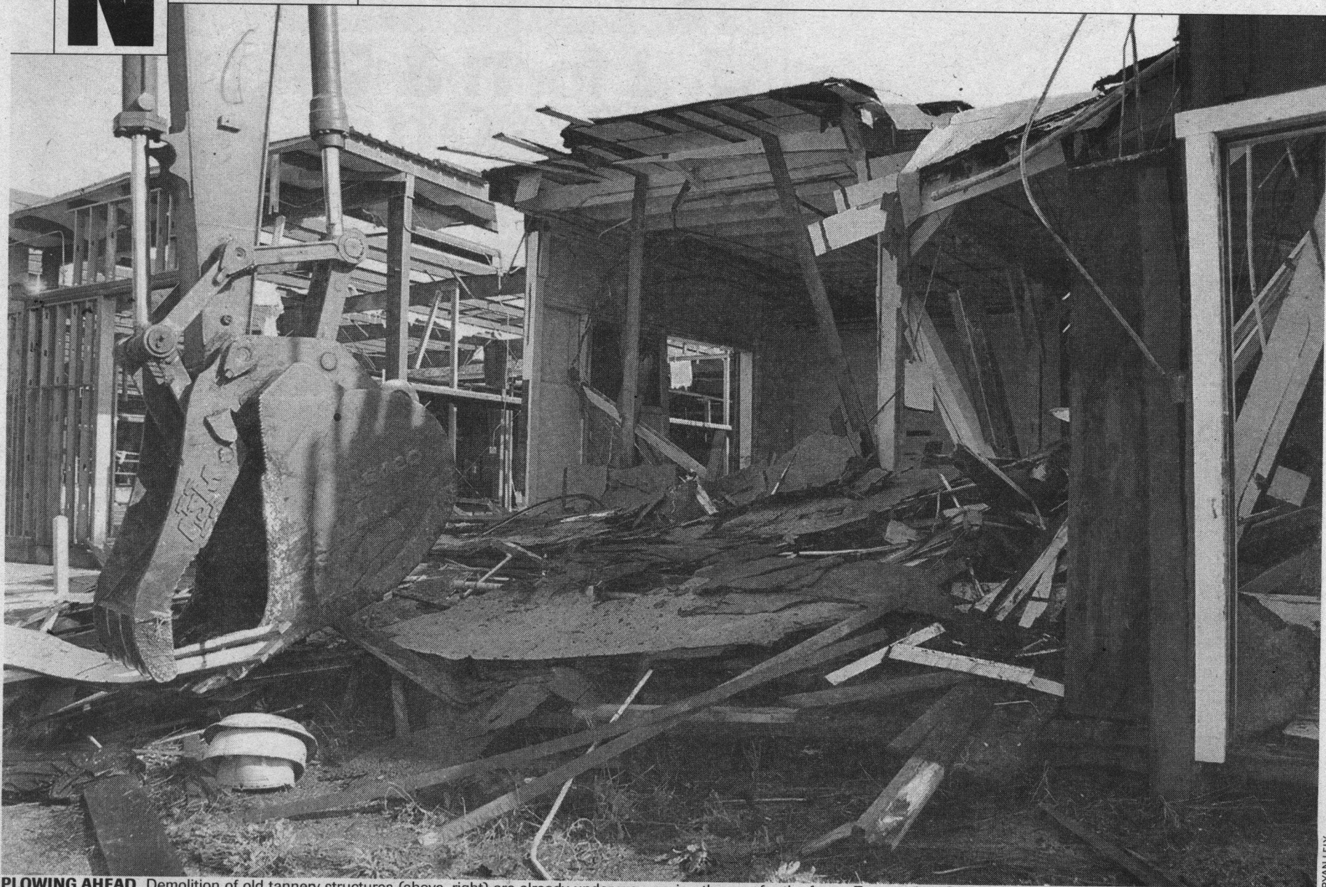
PLOWING AHEAD Demolition of old tannery structures (above, right) are already under way, paving the way for the future Tannery Arts Center.
