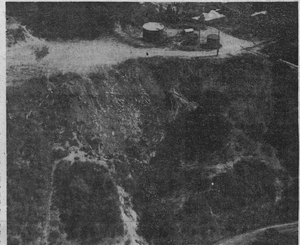
The big 50,000-gallon storage tank pictured here is a sore spot with the people who think the Central Santa Cruz County Water District is leading them down the tire-strewn brimstone path. They think the erosion is a shame in the first place, and that the tires and rubble which
