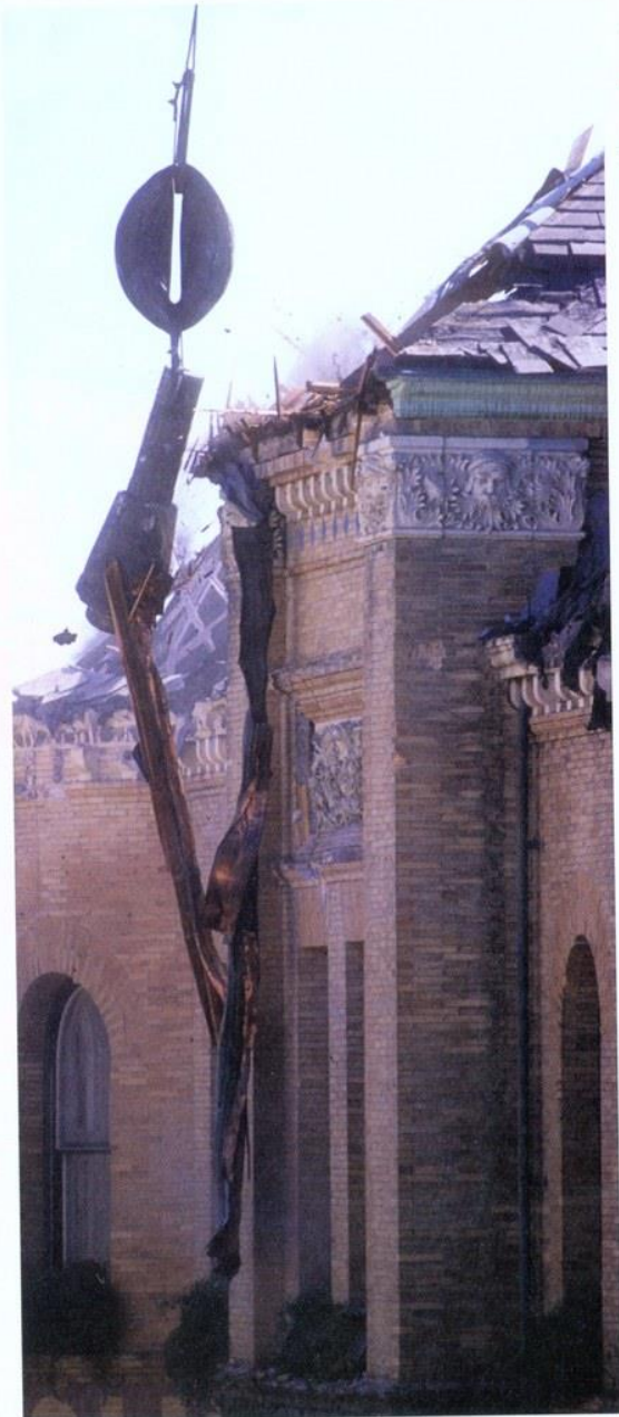
(Above) Although building contractor Michael Bates had recently completed an earthquake retrofit and the building sustained very little damage, hundreds watched as the beloved Cooper House fell victim to the wrecking ball. Spectators gasped as the ball struck three times before doing any damage.
